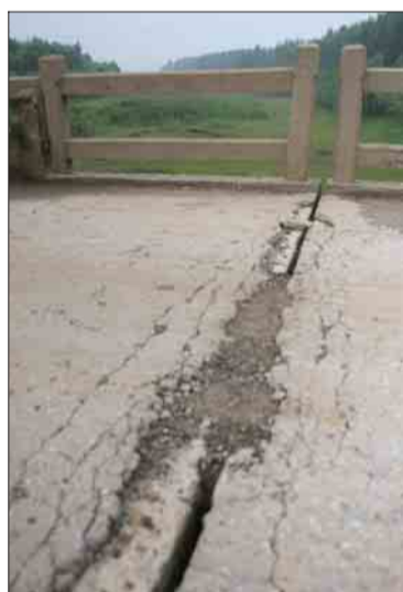
Cracks in the bridge in Hebei province where Wang Bingliang died last April. Photos: Lulu Chen
